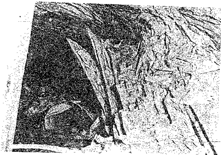
Figure 113 : Collapse of a mine haulage under severe rockburst conditions in a deep level gold mine in South Africa.
