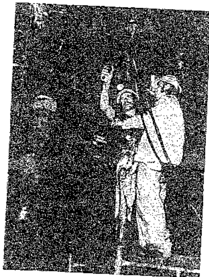
Figure 153 : Grouting a stressed 20m long high tensile steel cable in a slope back at the New Broken Hill Consolidated Ltd. mine.
