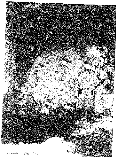
Figure 151 - Pre-reinforced drawpoint in a mechanised mine. Reinforcing bars were grouted in place, as illustrated in Figure 149, during development of the drawpoint and before the ore was blasted. Excellent stability was achieved in this example.
