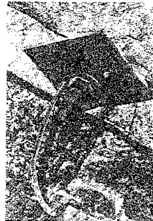
Installation of a rockbolt washer across the "sawtooth" profile of a blocky rock face makes subsequent sealing of the hole difficult.
