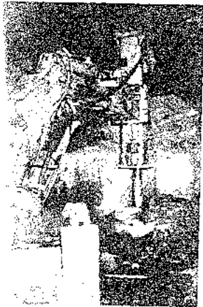
Heavy hydraulic hammer fitted to the articulated arm of a lift vehicle being used to scale boulders in a cavity. A range of equipment is used to assist manual scaling in hard constructions.
