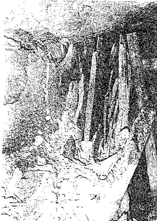
Figure 117 : Severe sidewall spalling in an excavation in quartzite in a deep level South African gold mine.
