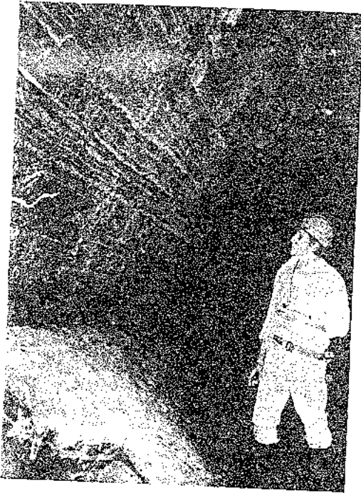
Figure 98 : Sidewall failure in a mine haulage designed parallel to the strike direction of two major discontinuities.
