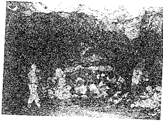
Figure 150 - Failure of a drawpoint brow in a mechanised mine resulting in loss of control of the process of drawing the broken ore. No reinforcement had been placed before the ore was blasted and attempts to reinforce the drawpoint brow with a steel beam set in concrete were not successful.
