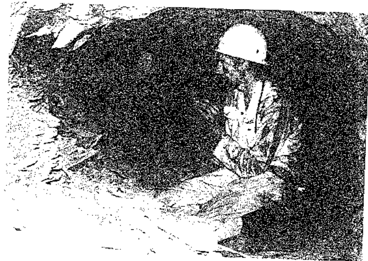
Figure 112 : Sidewall failure in a mine tunnel in very highly stressed rock in a mine in Zambia.
