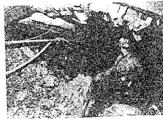
Figure 132 : Use of heavy steel sets in an attempt to control fracturing around a mine tunnel subjected to high stresses. The steel sets are too stiff for this application and cannot accommodate the deformation to which they are subjected.
