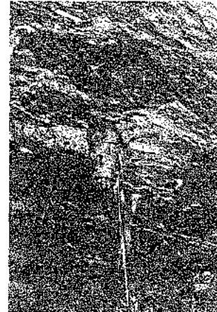
Stressed end of a 20m long grouted high tensile steel cable used for cut and fill slope back support at the New Broken Hill Consolidated Ltd. mine in Australia.
