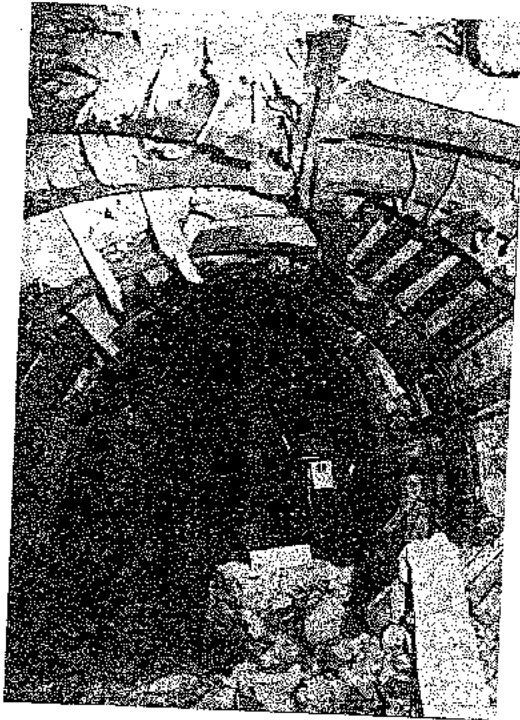
Figure 145 : Deformed steel sets providing support for a critical access tunnel in very poor quality rock under high stress.
