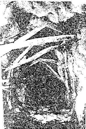
1. A portion of the same deformation indicated by the buckled and spalling of this mine tunnel has been controlled by the application of a thin concrete layer and stability is adequate for temporary access.
