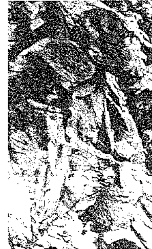
The sad remains of what could have been a perfectly safe and stable rock face.
