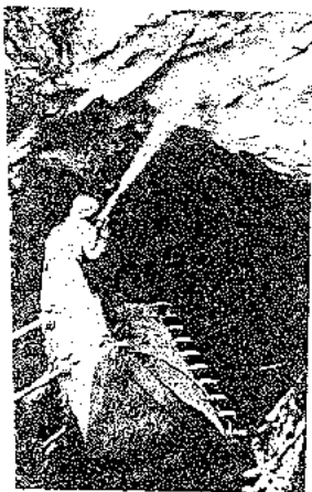
Success of a shotcrete operation depends very heavily upon skill of the nozzleman.
