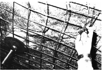
Welded wire mesh, firmly attached to the rock surface, provides excellent reinforcement for shotcrete.
