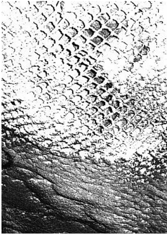
Chainlink mesh, while very strong and flexible, is not ideal for shotcrete application because it is difficult for the shotcrete to penetrate the mesh.
