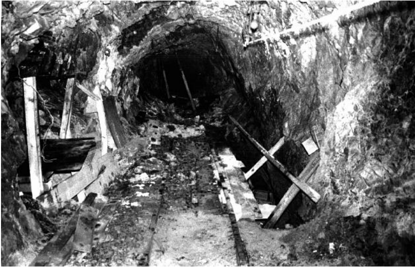
Figure 11.3: An accumulation of small blocks and wedges which have fallen from the roof and walls of an unsupported tunnel in a closely jointed rock mass. These small failures, induced by mining activities in adjacent stopes, could be controlled by the installation of light support systems such as those illustrated in Figures 11.1 and 11.2. A layer of shotcrete can provide very effective support for this type of rock mass.
