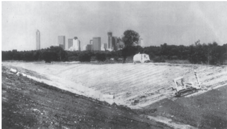
Figure 13.23 Slope stabilization of a canal bank by pressure injection of lime–fly-ash slurry (Courtesy of Hayward Baker Inc., Odenton, Maryland.)
