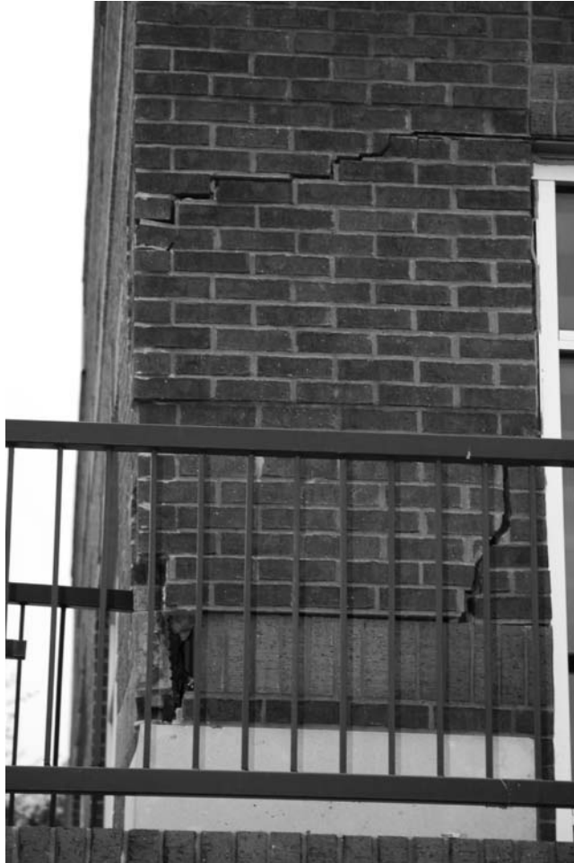
Figure 13.8 Cracks in a wall due to heaving of an expansive clay (Courtesy of Anand Puppala, University of Texas at Arlington, Arlington, Texas)
