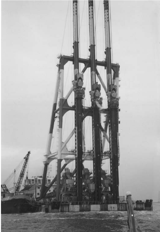
Figure 14.36 Construction of sand compaction pile in Yokohama, Japan Harbor (Courtesy of E. C. Shin, University of Incheon, Korea)
