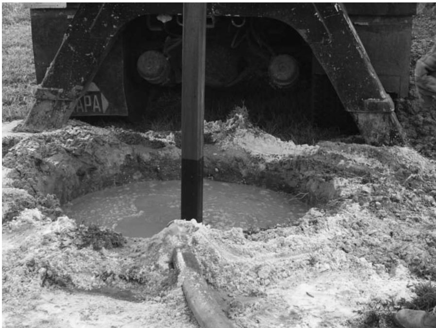
Figure 12.6 Drilled shaft construction using wet method (Courtesy of Khaled Sobhan, Florida Atlantic University, Boca Raton, Florida)
