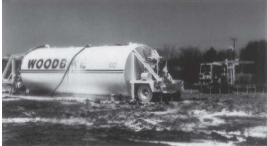
Figure 13.22 Pressure injection of lime slurry for a building pad (Courtesy of Hayward Baker Inc., Odenton, Maryland.)
