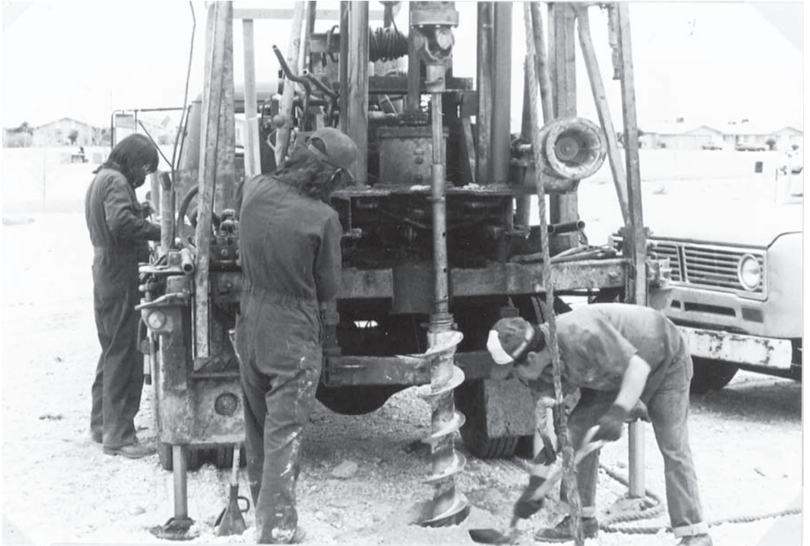
Figure 2.12 Drilling with continuous-flight augers (Danny R. Anderson, PE of Professional Service Industries, Inc, El Paso, Texas.)
