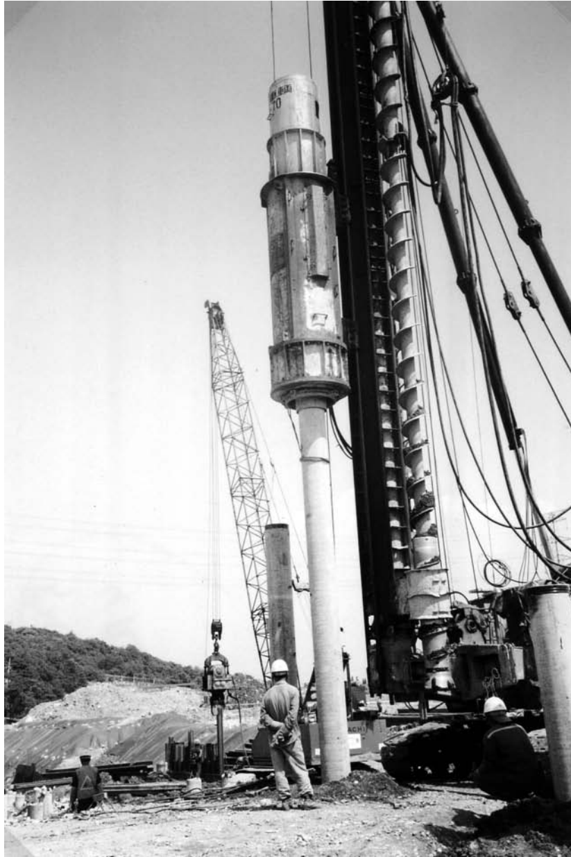
Figure 11.8 A pile-driving operation in the field (Courtesy of E. C. Shin, University of Incheon, Korea)
