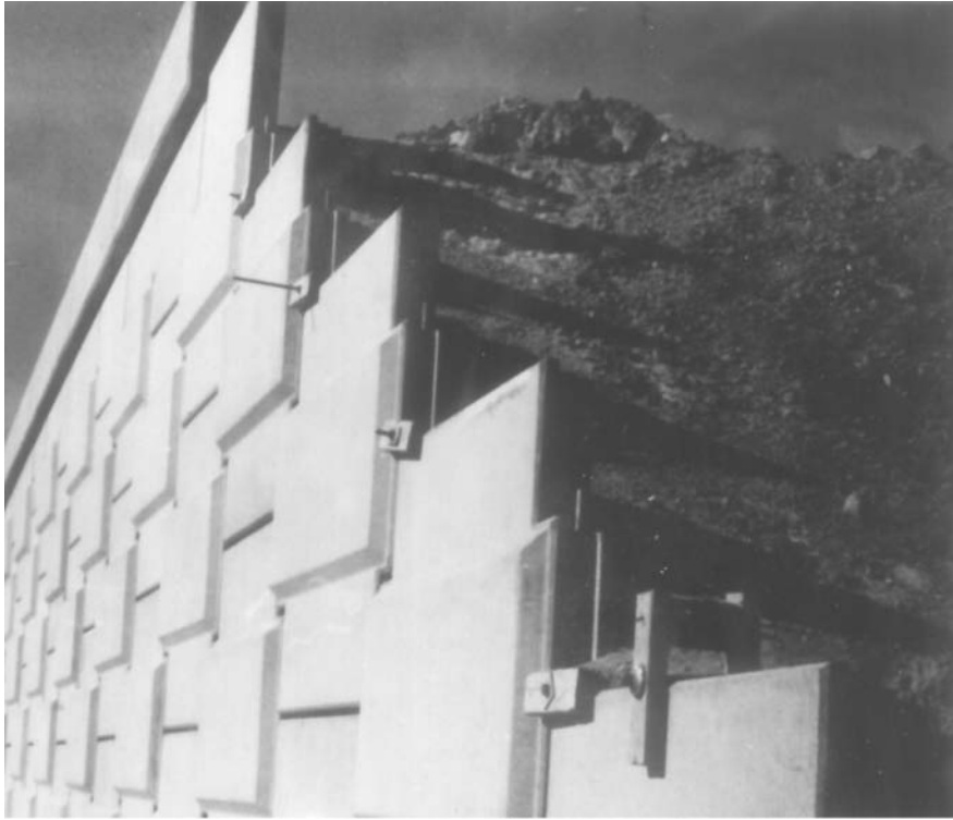
Figure 8.27 Another view of the retaining wall shown in Figure 8.26 (Courtesy of Braja M. Das, Henderson, NV)
