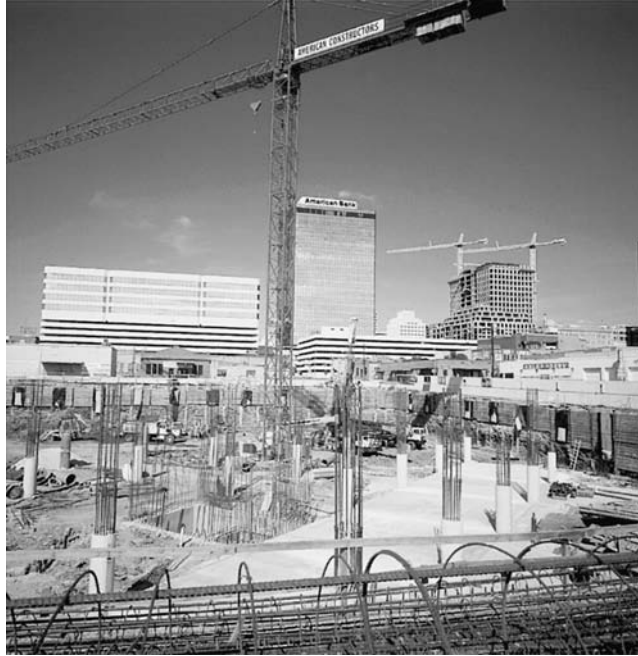
FIGURE 13.1 Concrete piles used for the foundation of a skyscraper. (© Fritz Henle/Photo Researchers.)
