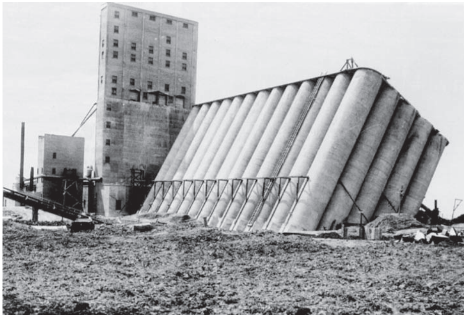
FIGURE 1.6 Failure of the Transcona Grain Elevator. (Photo courtesy of Parrish and Heimbecker Limited.)
