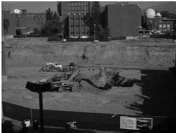
FIGURE 8.1 An excavation near a high-rise building. The applied loading history of soil elements at the same depth at the edge of the excavation and at, say, the center of the building will be different.
