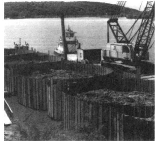
(b) Cofferdam under construction showing initial part of cell line 1-2 with cells being partially filled for stability.
