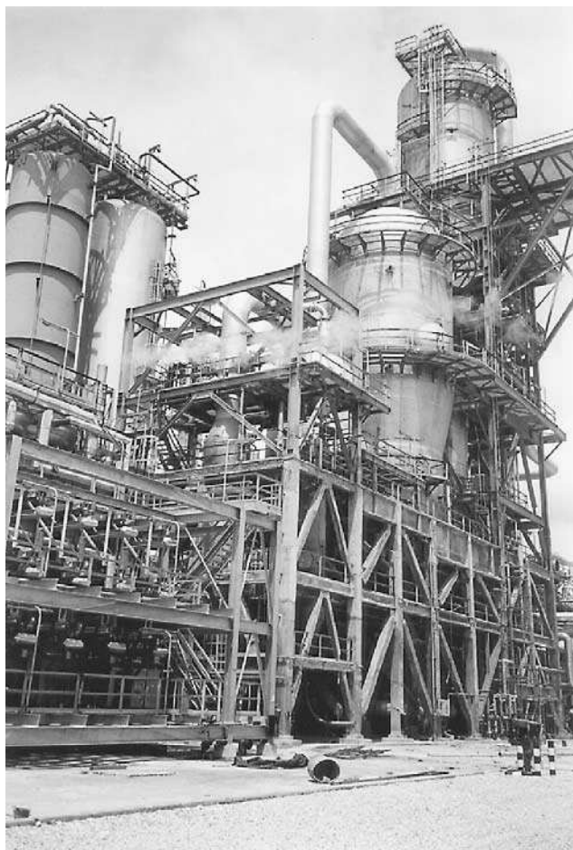
FIGURE 3.2.1 DCC unit at TPI refinery, Thailand.
