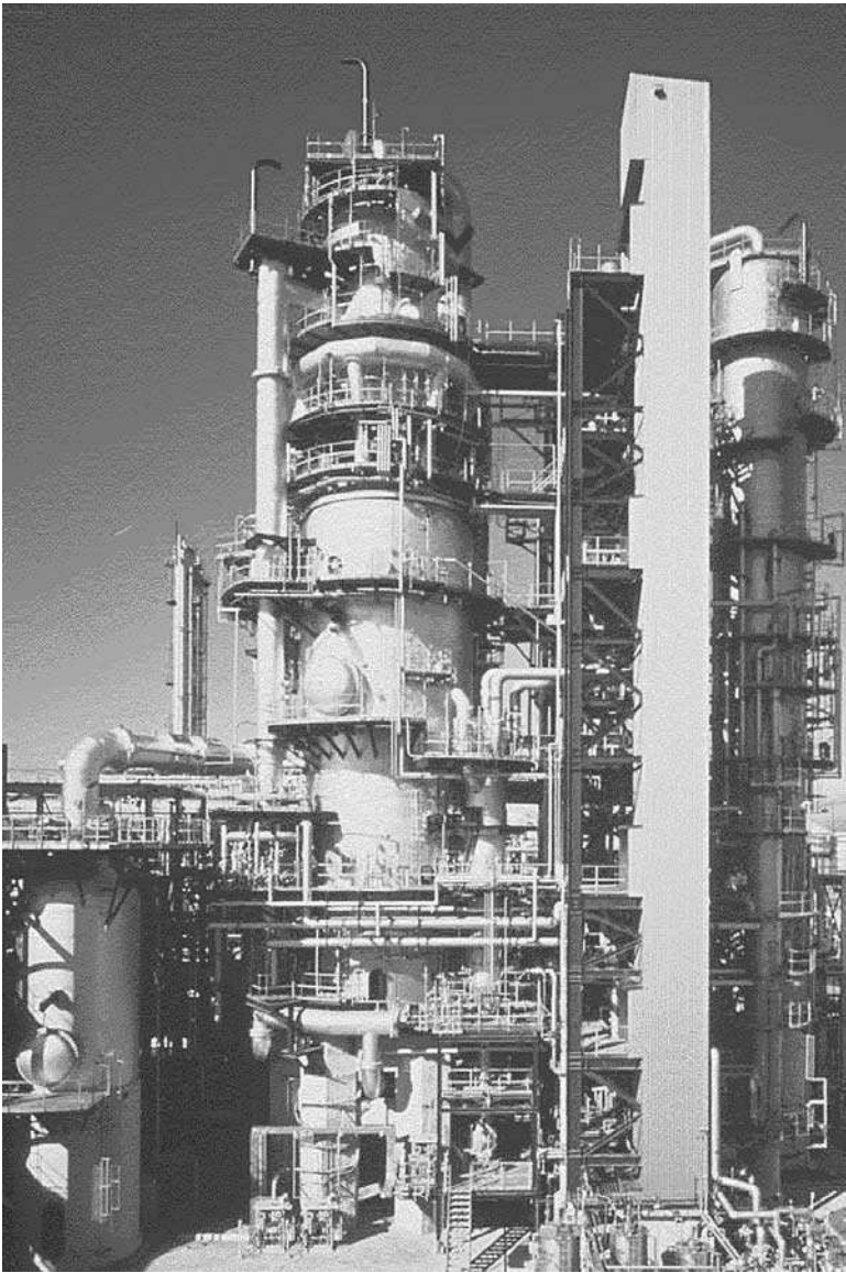
FIGURE 3.1.1 KBR Orthoflow FCC unit.
