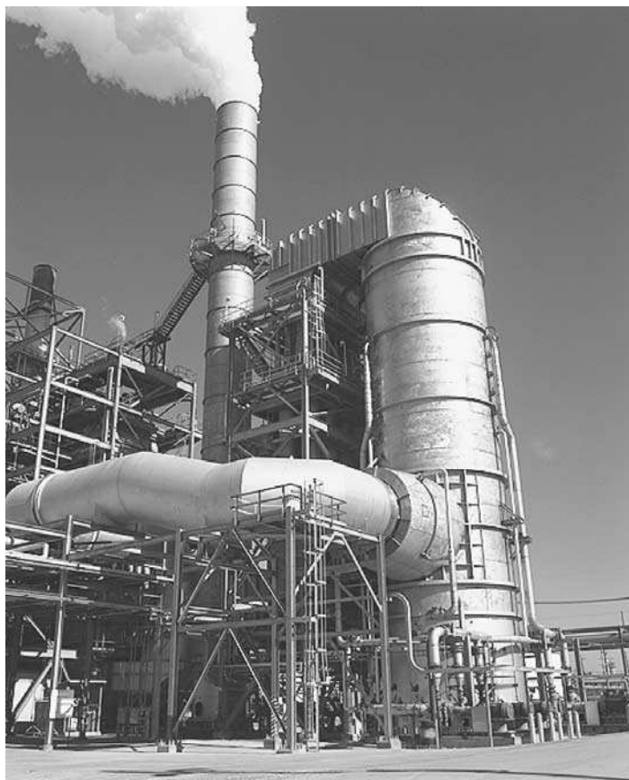
FIGURE 11.2.2 EDV wet scrubber at U.S. Gulf Coast refinery.
