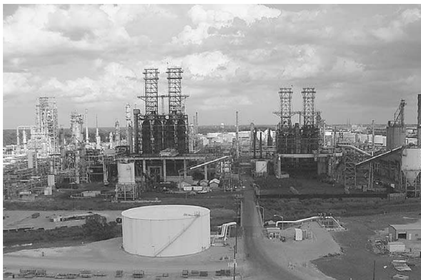
FIGURE 12.1.2 ConocoPhillips delayed cokers at Lake Charles, La. Structure on the left side of the photo is the fuel-grade coker. On the right is the premium coking unit.
